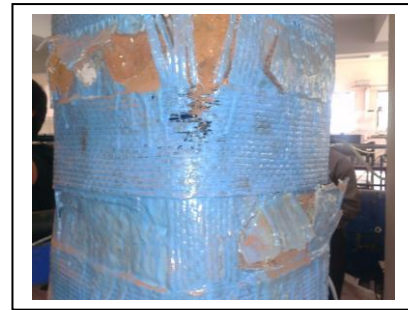
Figure 6 : Failure of CWOA Specimen
